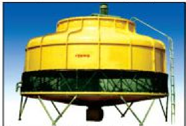
Cooling Tower at Shimanto Square (BGB)
