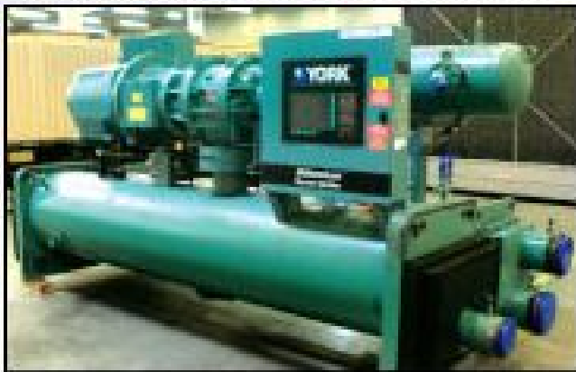
Pan Pacific Sonargaon Hotel, YORK Chiller
